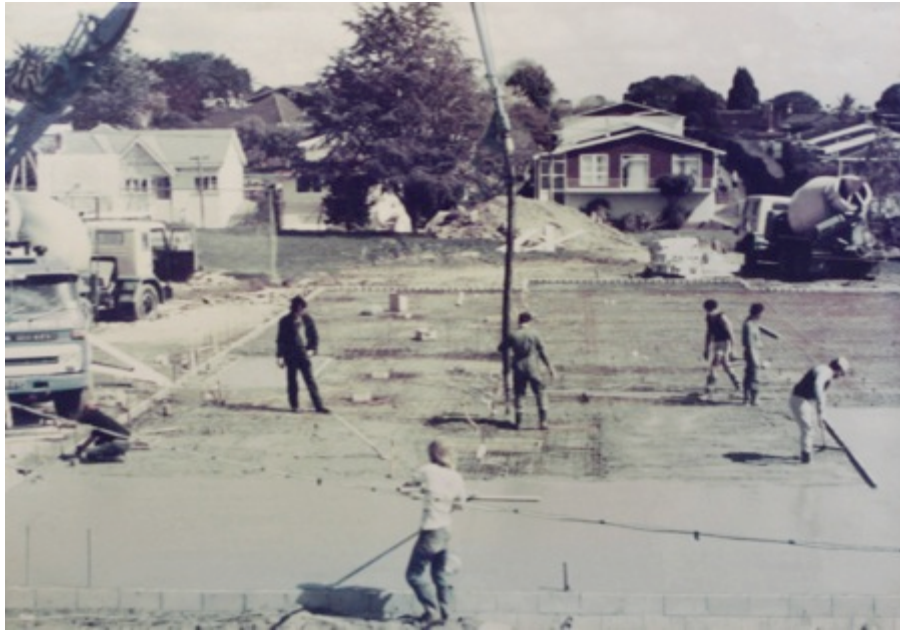
This image shows the slab being laid. In the background is a mature Himalayan cedar ( Cedrus deodara ) on an extensive lawn. (Both were lost for a building commemorating a later jubilee).
