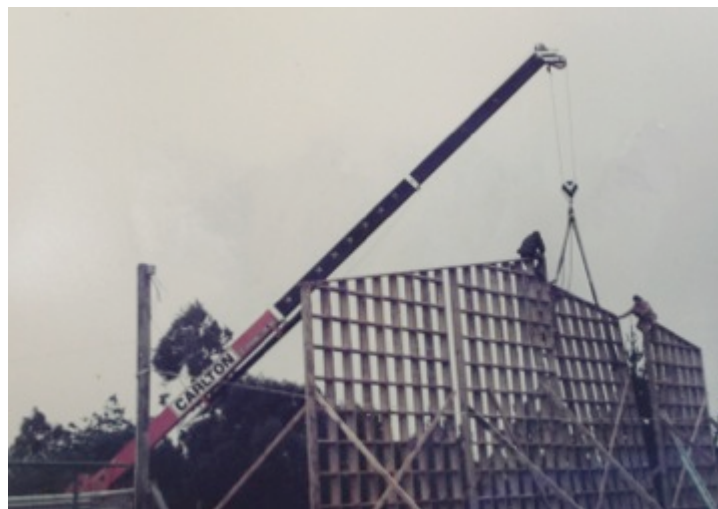
This photograph shows a large section of prefabricated framing at one end of the building being craned into place. Although not clearly visible it appears that the workmen atop the framing have vests with lines attached to the crane.
